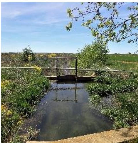
There were these irrigation systems all along the way.
